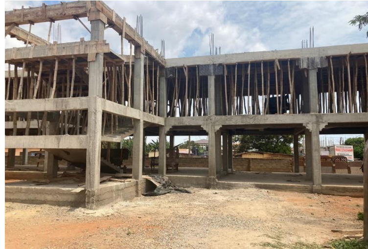
CONSTRUCTION OF 2 STOREY CLASSROOM BLOCK AT AL-RIYAAD BASIC SCHOOL (PHASE I COMPLETED)
